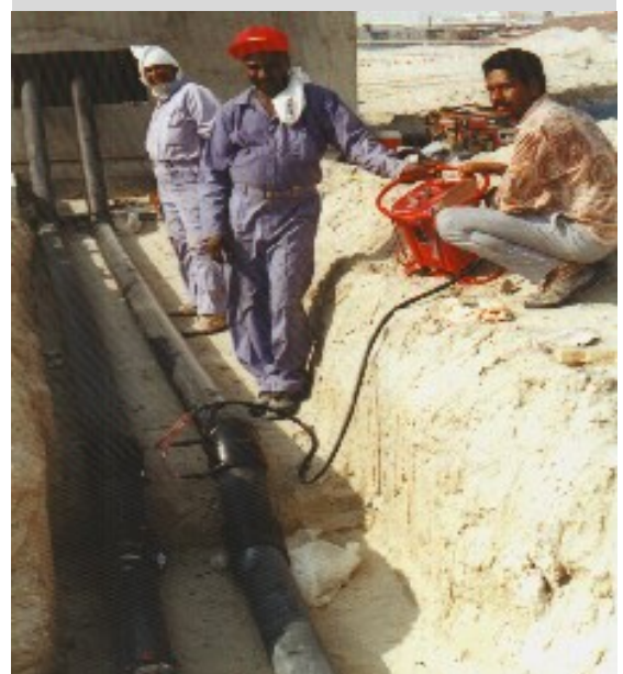
Shallow vacuum pipework entering station
